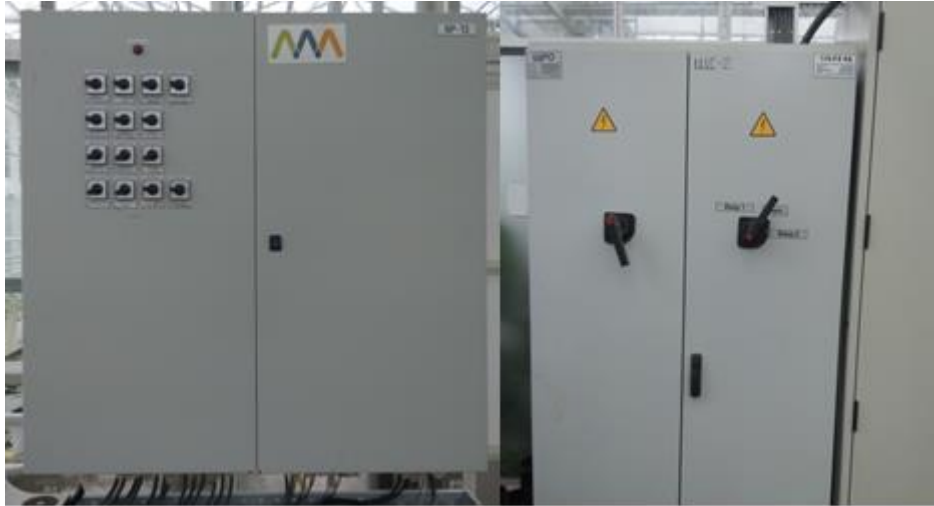
Figure 23. Electrical panels: a) control panel section; b) the distribution board.
