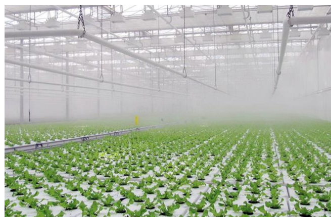
Figure 7. Fog irrigation system
