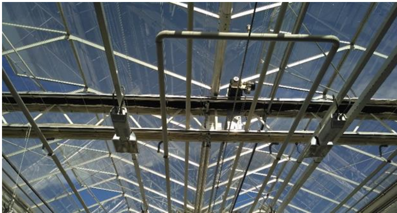
Figure 14. Ventilation system (transoms).
