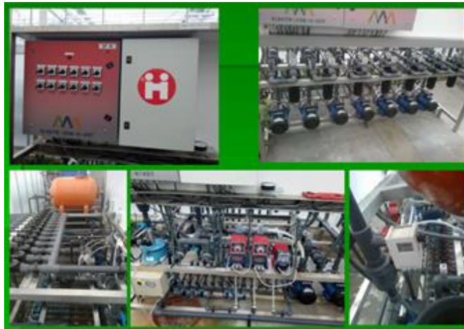
Figure 24. The control system of irrigation.
